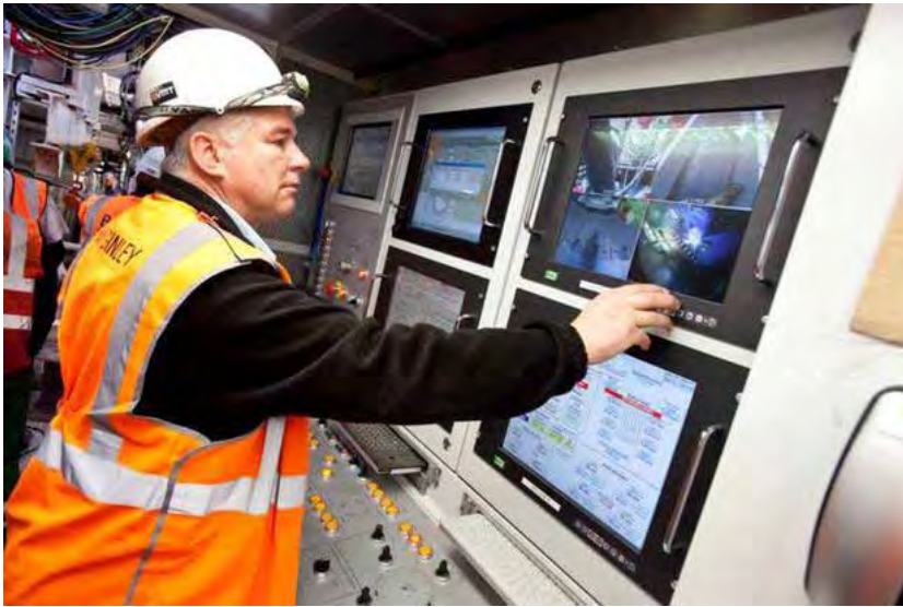
Control: the operations room for Crossrail's giant tunnel boring machine (TBM), Phyllis
