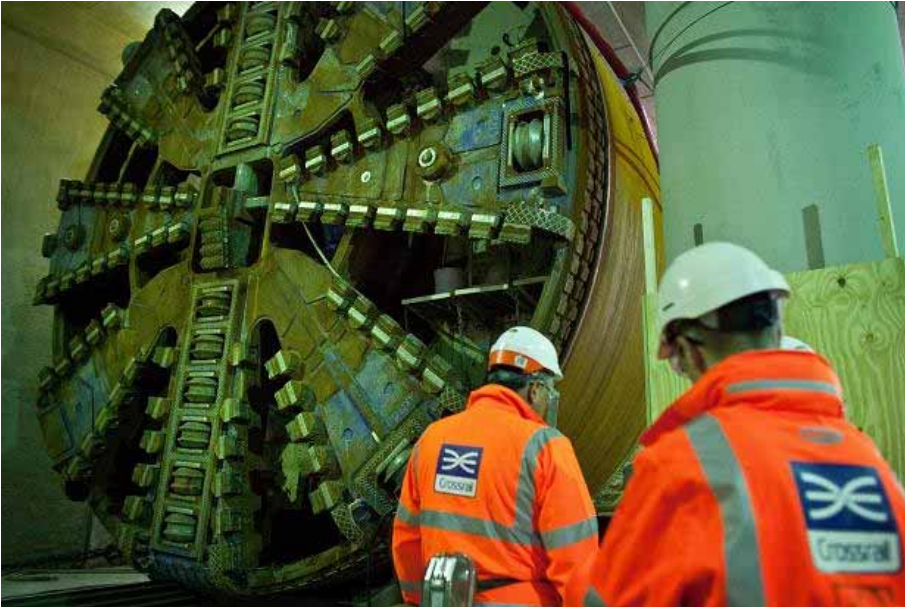
Tunnel vision: The Crossrail scheme is on track but its chief executive is warning of a future talent drain abroad Times photographer, Ben Gurr
